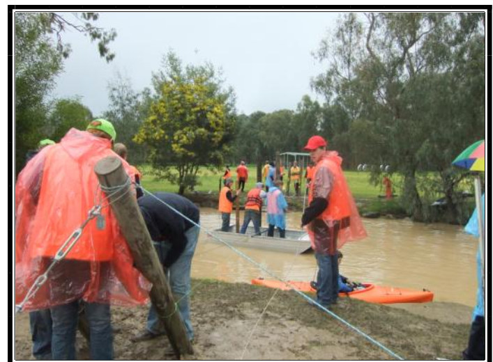
Build A Bridge—Day three. Despite the wet weather construction of the full scale bridge began on time
